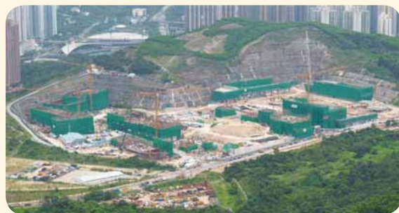
● 興建中的新消防訓練學校工程進度理想 Construction works of the new Fire Services Training School are in good progress
